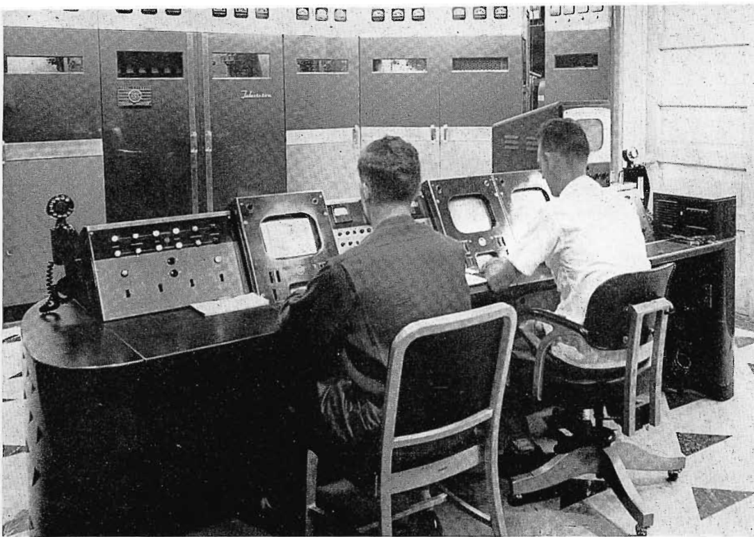
FIG. 24. KMTV uses an RCA TT-5A 5-kw VHF transmitter with a TT-25AL amplifier.
